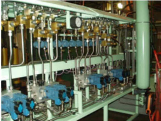
Figure 11. The new upgraded valve panel included close isolation valves and additional safety features.
