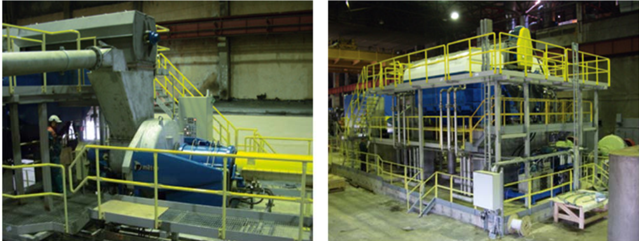
Figure 10. An RGP 262 refiner fed by a TRPW-1532 twin roll dewatering press provided good stock preparation before the Valmet Breast Roll Shaker unit.
