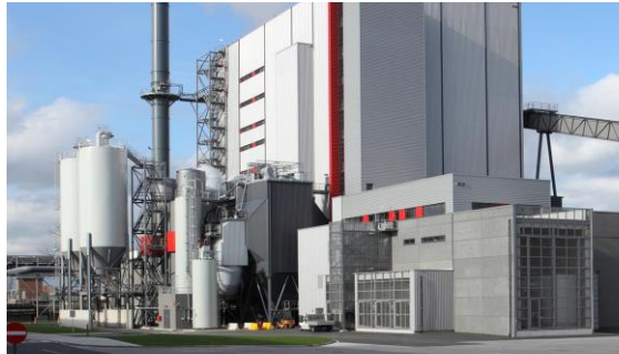
Valmet's CYMIC boiler at Stora Enso Langerbrugge
